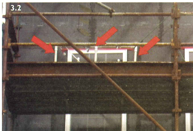
Figure 3.2: Qualitative water testing of window and stud wall assembly after installation of membrane water proofing. Note spray rack (red arrows) above and to the side of window that washes the wall while the cavity side of sheathing is checked for leaks. Figure 3.3: Checklists for commissioning of sliding glass doors. These checklists are completed by the contractor. The checklists may be modified after installation and quantitative testing of the first several doors.
